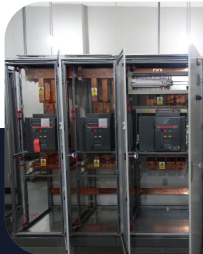
Main Distribution Board (MDB)
