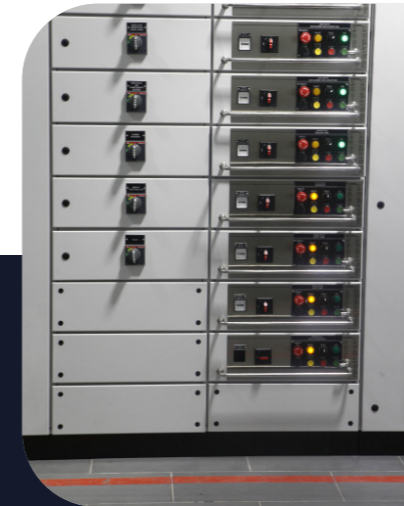
Motor Control Center (MCC)
