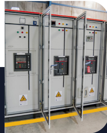
Automatic Transfer Switch (ATS)
