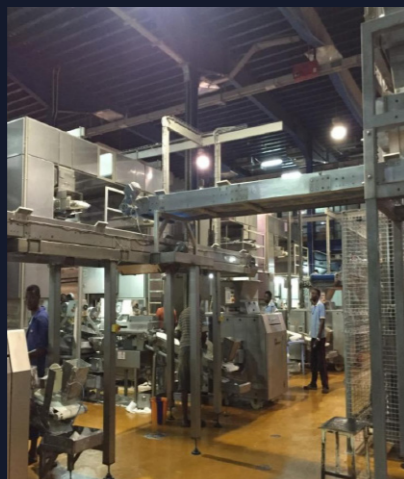
FACTORY PAIN VICTOIRE-KINSHASA Lighting Installation, Small Power, Bust Duct System, Electrical Power Plant, Transformer, Generator, Main & Sub- Main Distribution Panel Boards.
